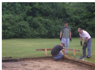
Greg Reed, Thad Hallberg, and David Rousse (L to R) lay a firm foundation for the new outdoor performance pavilion.
